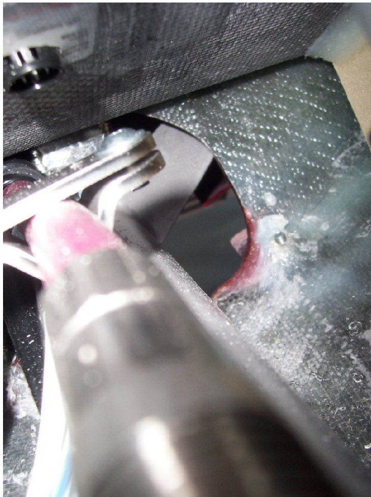
Fig 5 View aft showing clamp fitted underneath grommet
